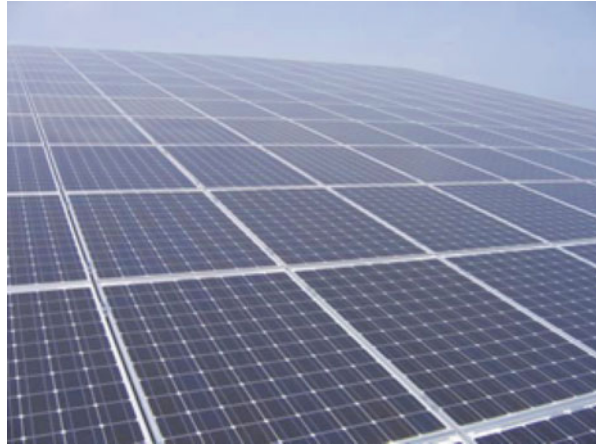
Fig. 8.2 300 m 2 , 29.7 kWp PV installation producing about 10 % of my practice energy (30 MWh/year)
