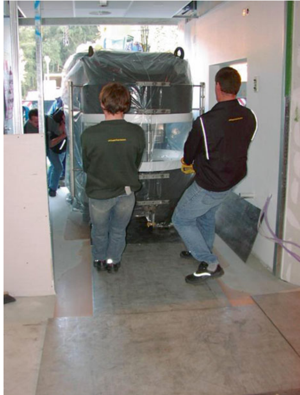
Fig. 3.3 Installation of a 0.35 T magnet (Siemens Magnetom C!, Siemens Healthcare, Germany). Important: protection of the floor by steel plates
